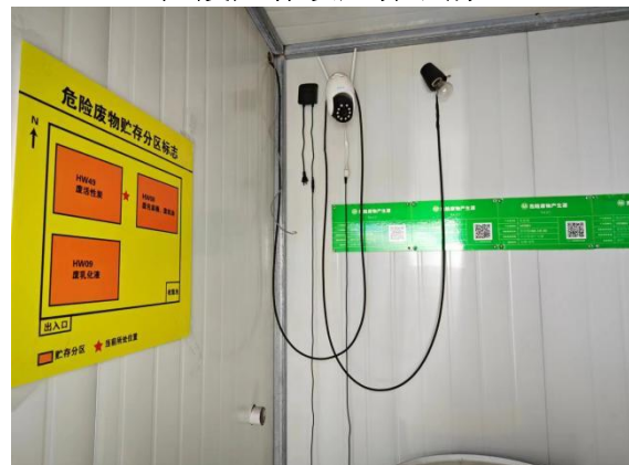
危废仓库废气收集口及内部危废标牌
